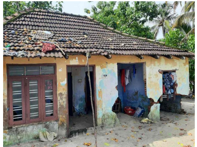
Pic 12: Houses of Rajamma Das Veliyilparambu and Mollayil Nelson in Cheriyakadavu, destroyed in May 2021
