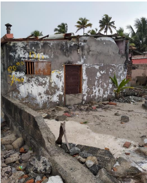
Pic 3: Another fully destroyed house in Chellanam
