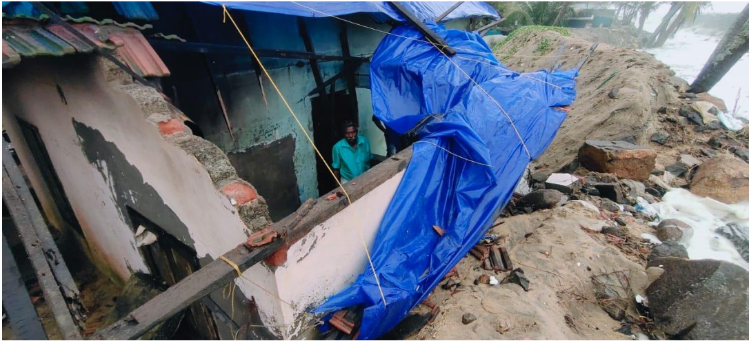
Pic 13: House being destroyed by large waves in Veliyathanparambu, Nayarambalam
