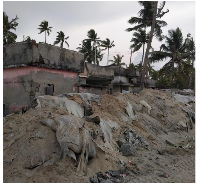
Pic 2: Geobags destroyed by sea water and mud in Chellanam
