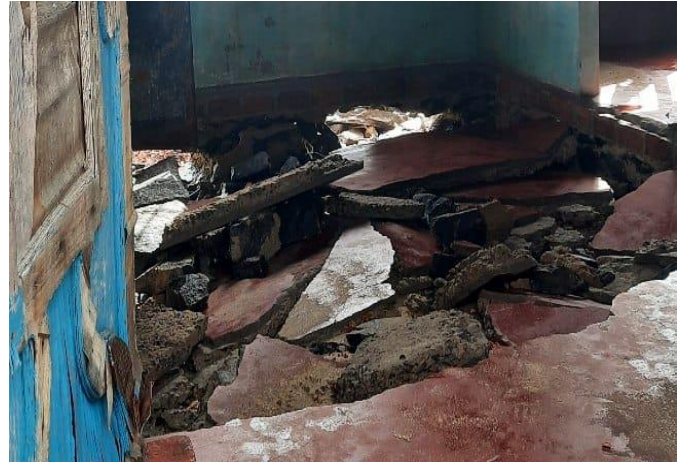
Pic 10: The inside of a house in ward 8 of Kannamaly. Sand deposits about a foot-high were formed here during the Tauktae cyclone in May 2021
