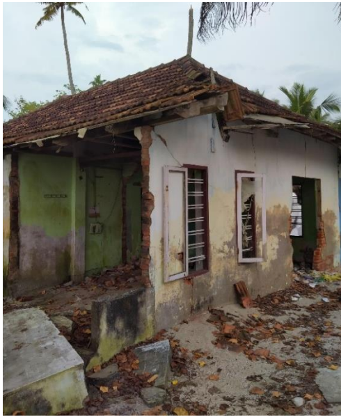
Pic 1: Damaged house in Velankanni, Chellanam
