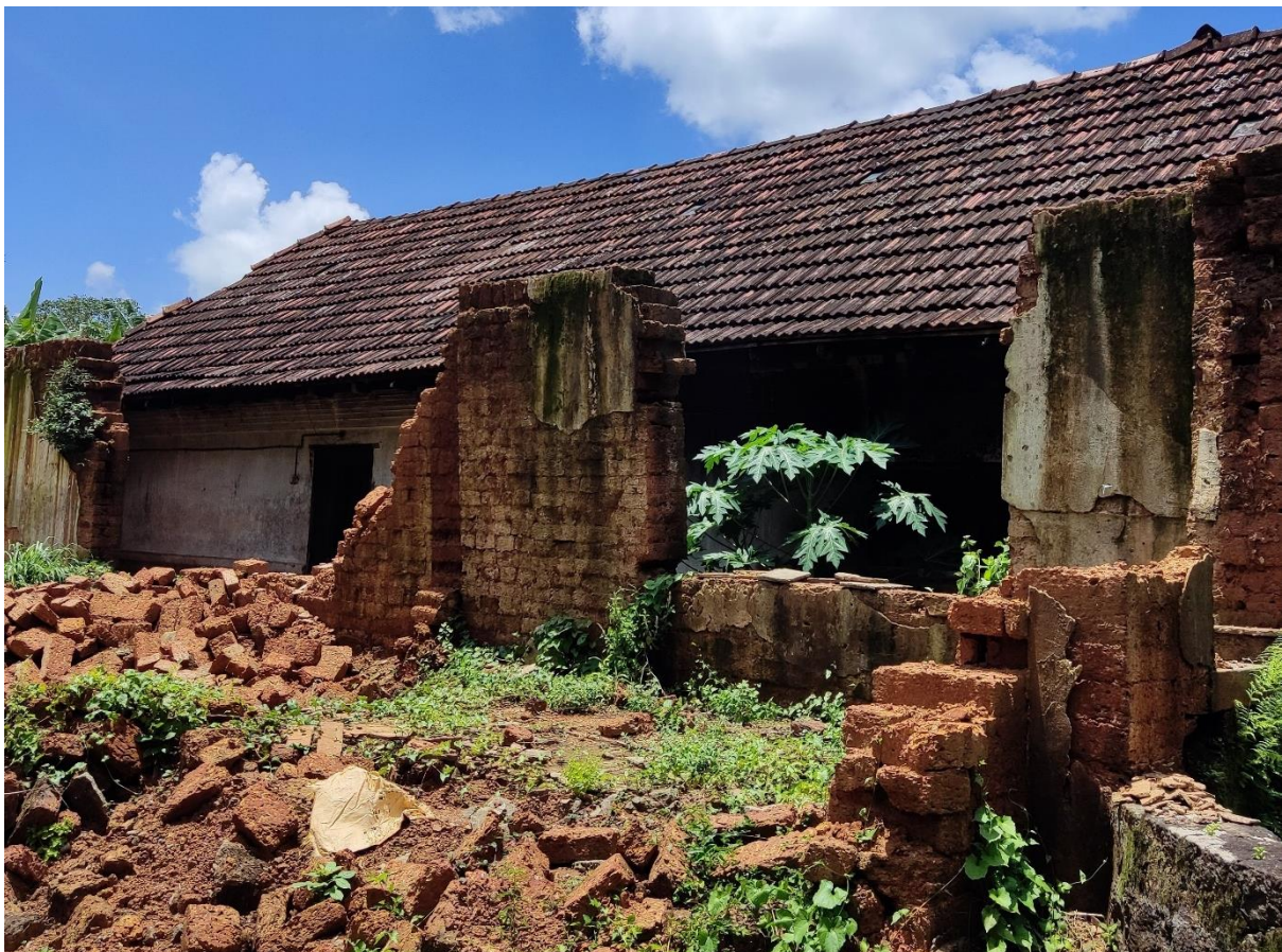
Pic 6. Dilaptated condition of the Mana
