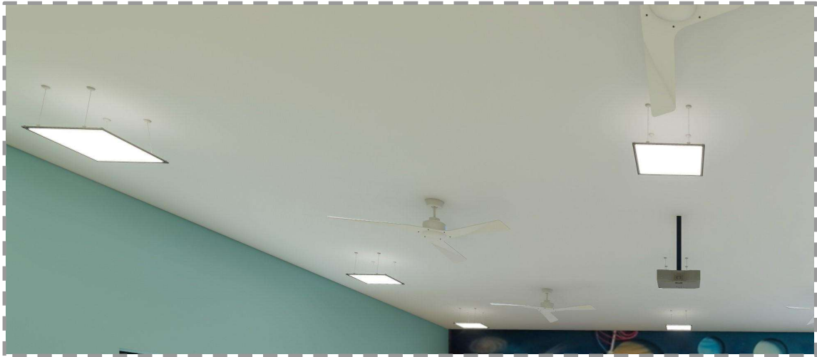
Plate 7: Lights and fans
